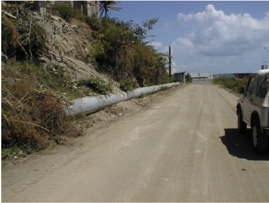
Figure A4-7. Molasses Pipeline to Port Basseterre (St. Kitts)
