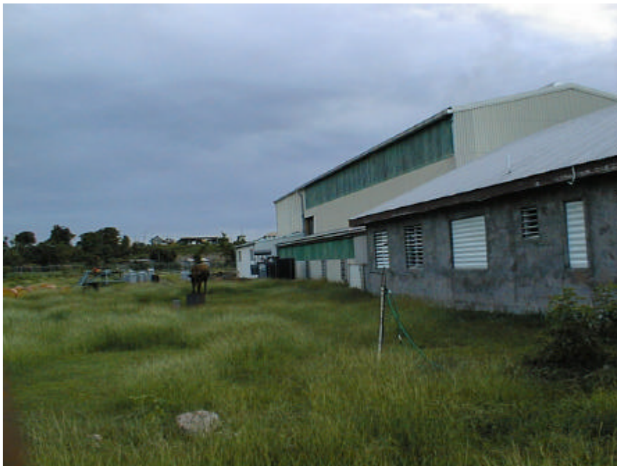
Figure A4-22. Power House (Nevis)
