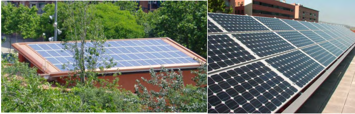
Figure 18- The photovoltaic modules installed on roofs have a high electricity production in Caribbean latitudes (versus PV on facades), besides, they reduce the thermal load from the ambient to the building if adequately ventilated
