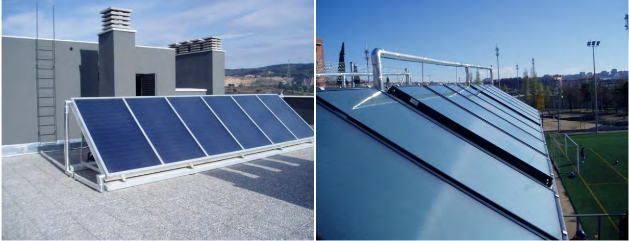
Figure 20- Service, commercial buildings (such as hotels, hospitals (right), sports centers (left) etc.) and residential buildings centralized solar thermal installations are the most effective solution to provide hot water all year round
