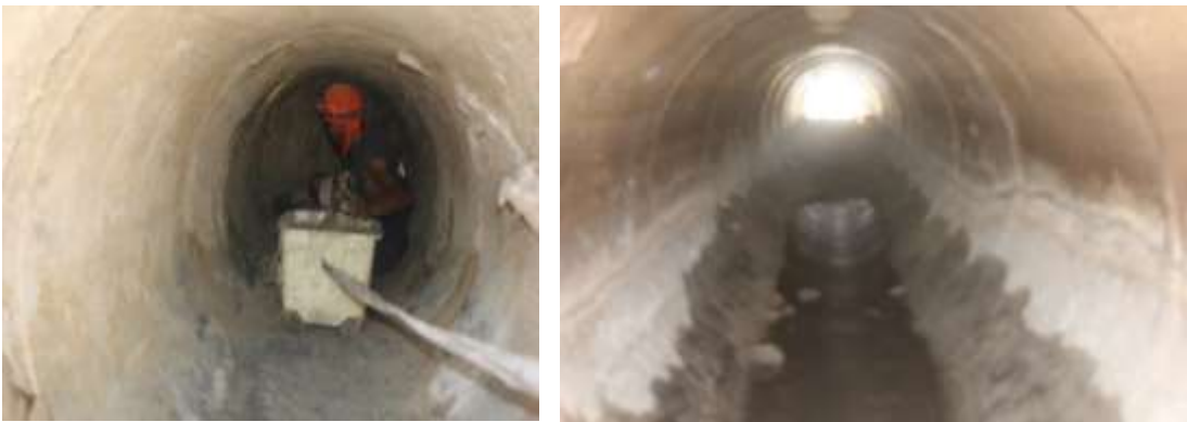
The inside of the drainage hole of the storm water drain. The picture on the left shows one of the manual labourer removing water filled, sand from the drain. The picture on the right shows the drain after complete clearance.
