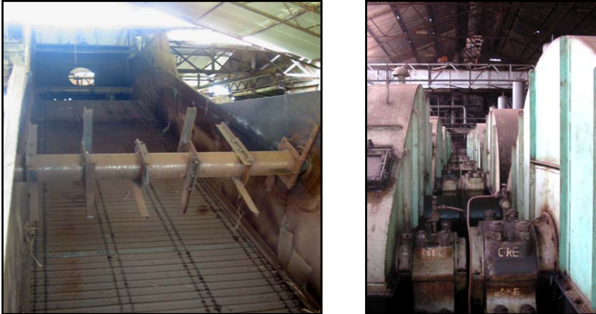
Figure 3.2. Conveyor Belt Entrance to SSMC Milling Facility (left) and the Five Installed Roller Mills at the SSMC (right)
