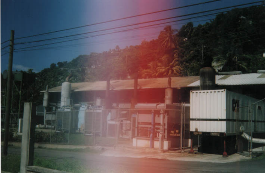
Figure A2-21. Major Diesel Generating Plant
