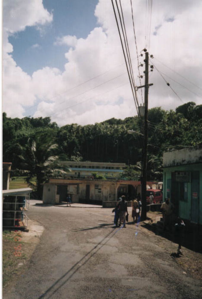
Figure A2-22. Electricity: High Voltage Pole/Lines (Low Voltage in Some Photos)
